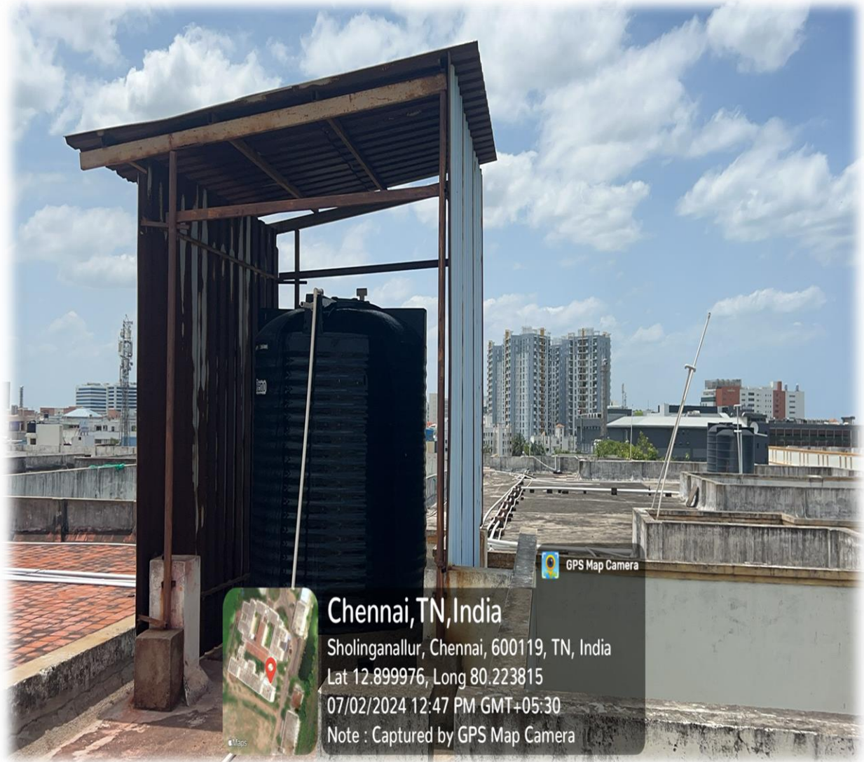
RO Water Tank @ Main Building
