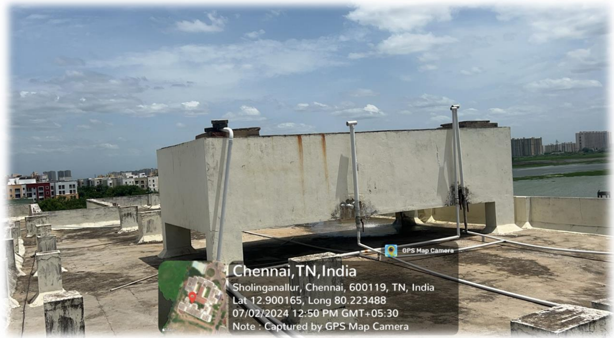
Recycled water tank @ Main Building
