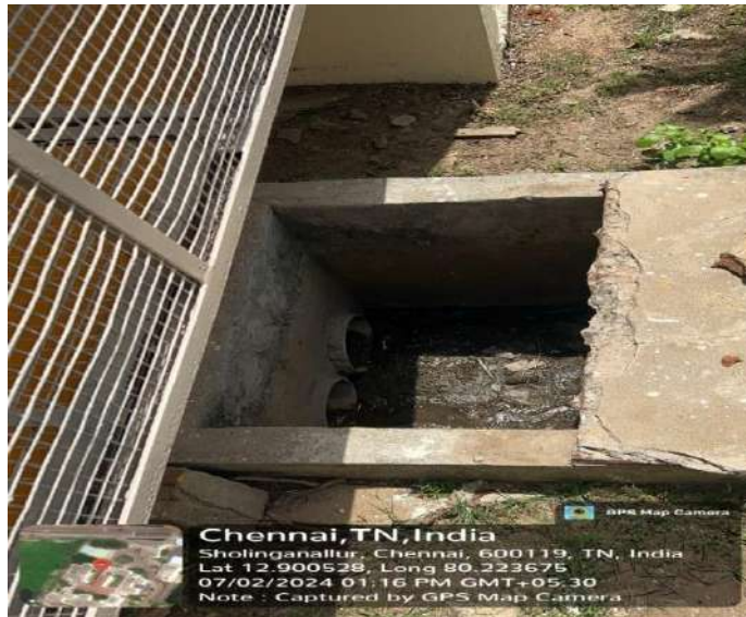
Rain water harvesting trenches pipe lines
